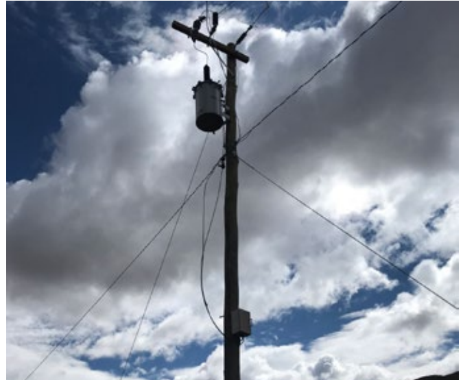
One out of over 200 poles that Johnson and other linemen help install in the Oruro region.
